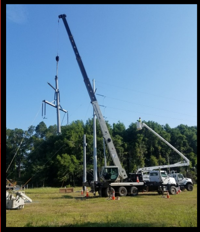
Building a bypass to isolate sub bays for rebuild at Archer Substation.
