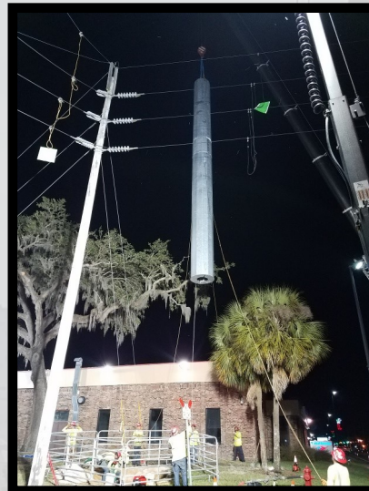
Working night shift due to traffic and outage constraints. Installing a self supported steel pole for line rebuild.
