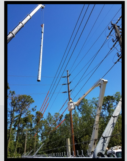
Changing out an angle dead end structure in Sebring, FL. Called in a sub contractor crane crew to set pole over existing lines.
